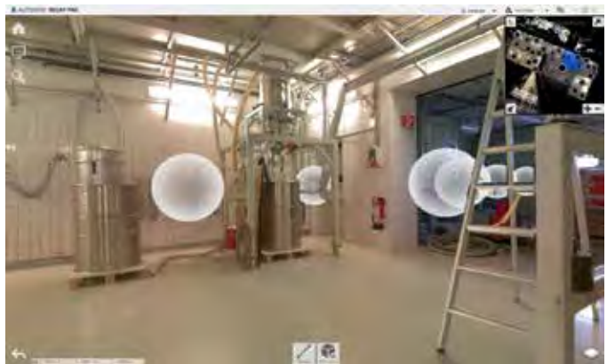
In addition to the point cloud, scanning also produces a complete image documentation with 360° images
