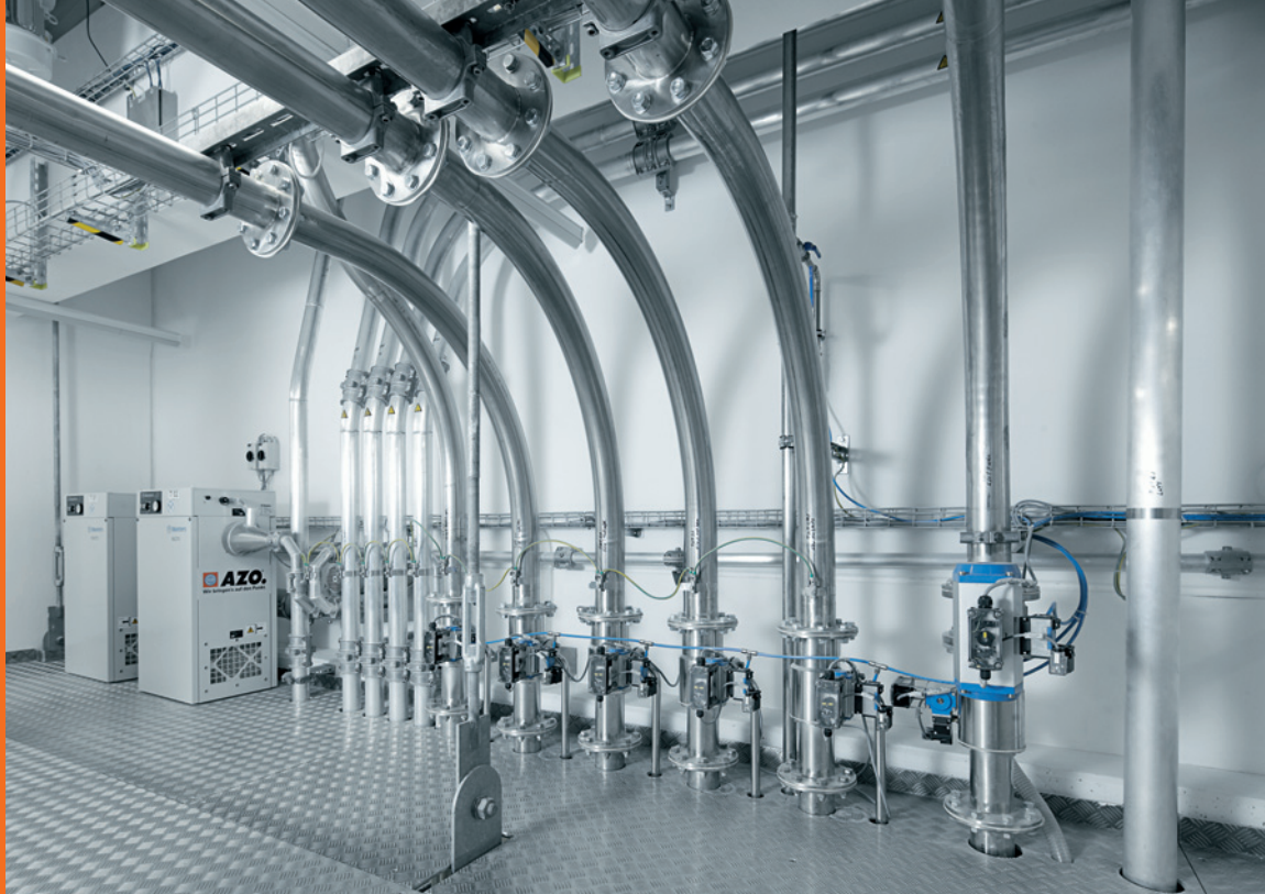
Silo fill lines and head room drying
