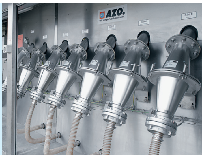
Silo head room drying and tank truck connections
