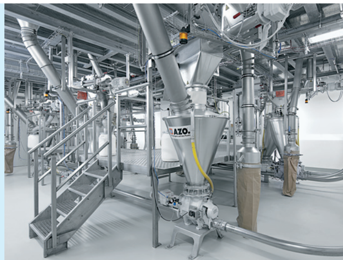
Cyclone screeners below the flour silos
