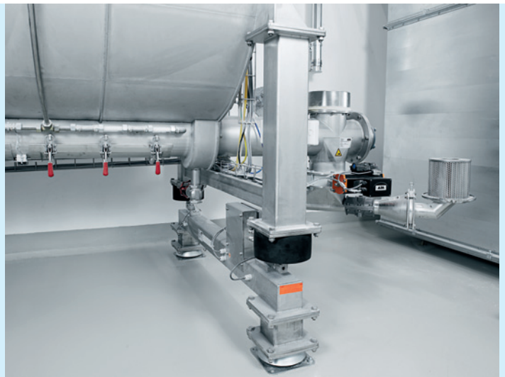
Hopper for powdered sugar on load cells with discharge screw conveyor
