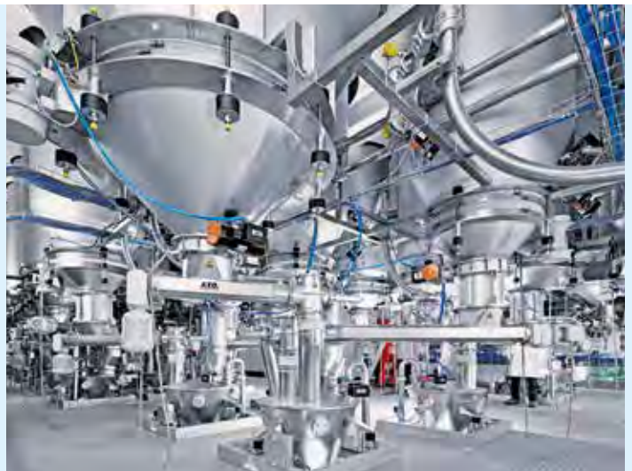
Discharge area for the salt silo with vibration bottoms and dosing screws
