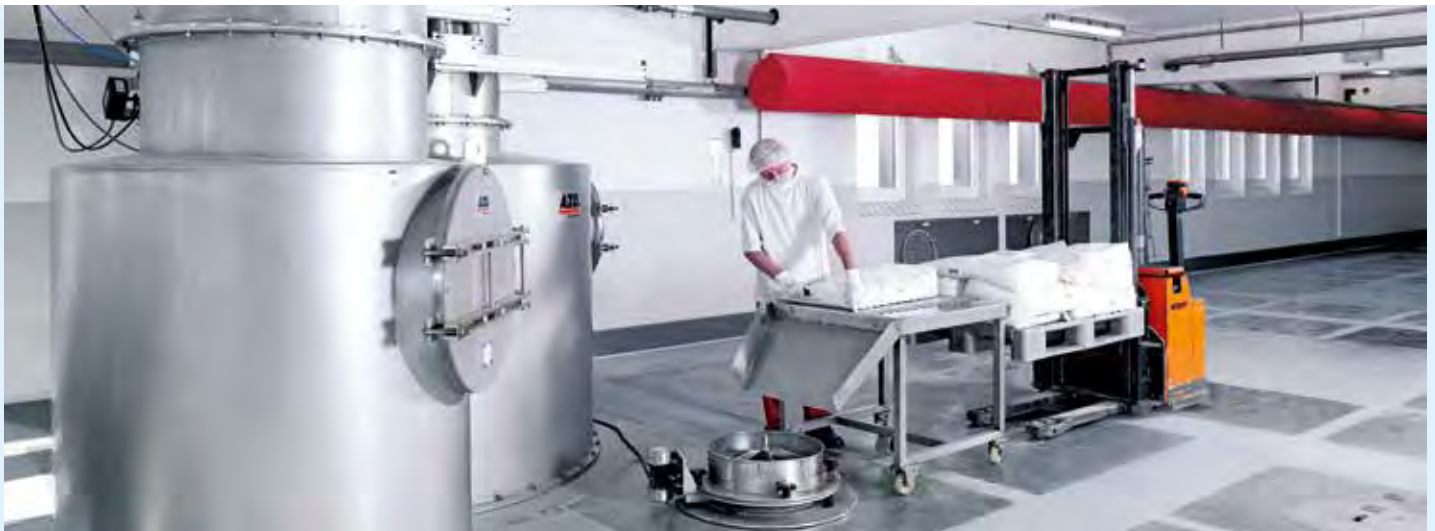
Filling the indoor silos with herbs from sacks via a vibrating perforated sheet
