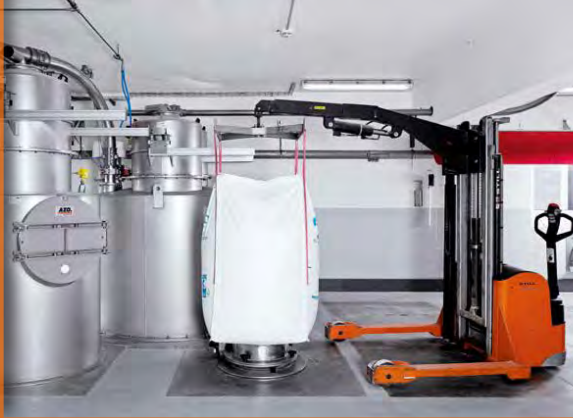
Big bags are discharged using a lifting device on account of the existing low storey height
