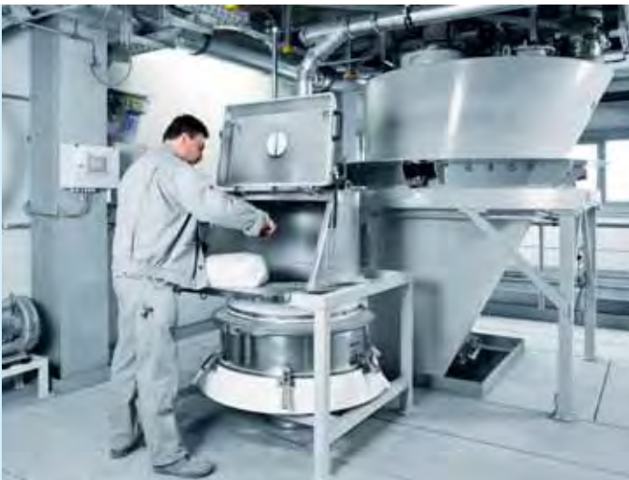
Scale hopper for premixes, pre-weighed raw materials are directly loaded into the mixer by means of a feeding hopper
