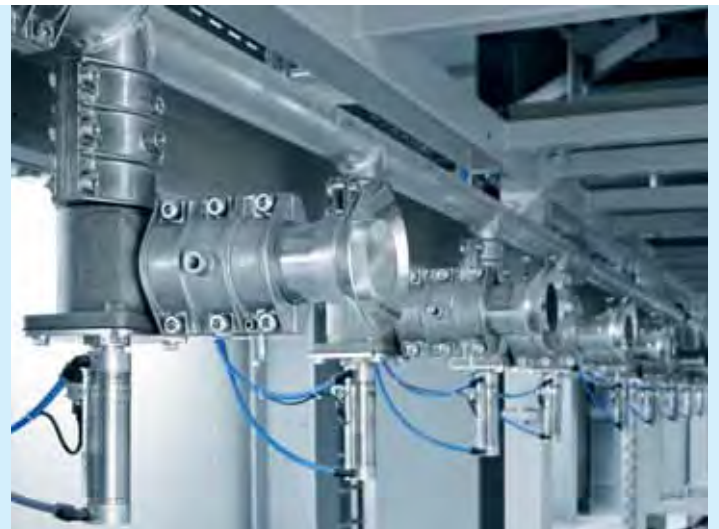
Automatic docking of the mobile scale hopper with the aspiration system
