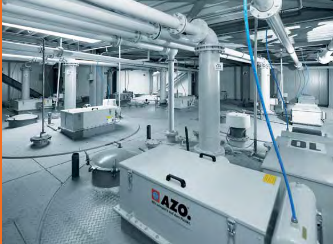
Bulk silos with filling lines and filters
