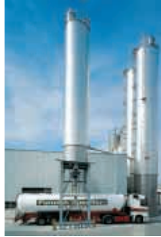
Loading of road tankers
