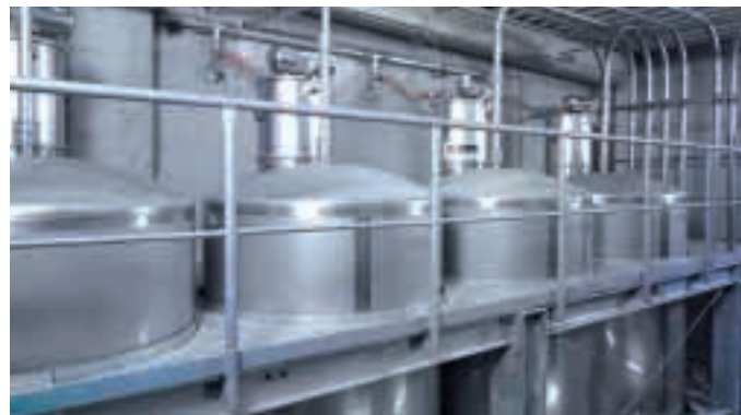
Buffer silos above the filling systems
