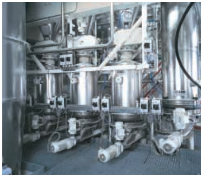
Buffer tanks with discharge and dosing system above the dosing level
