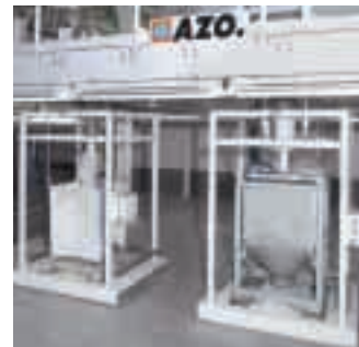
Filling of big bags and containers
