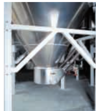
Outdoor silos with silo hopper connector
