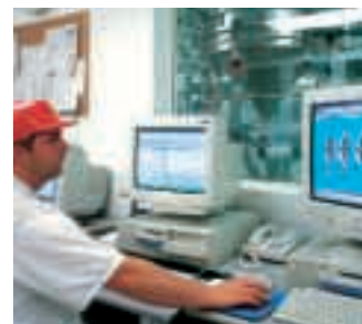
Central process control and visual display system
