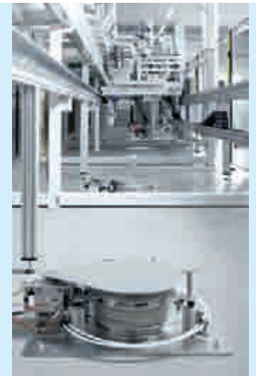
Supply point for pre-weighed batches
