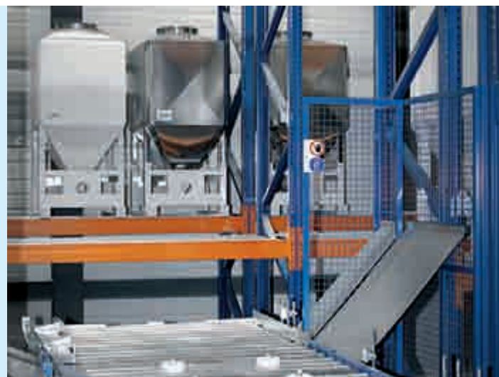
High-bay warehouse for the temporary storage of medium-sized and small components
