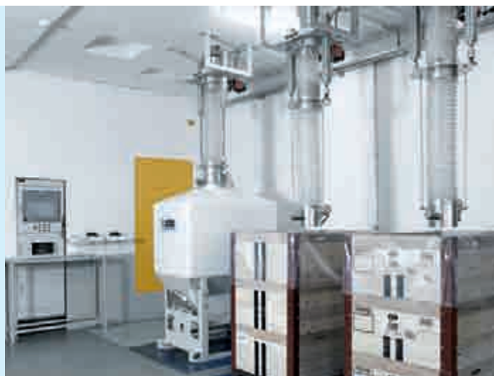
Operator terminal with barcode scanner in the finished product filling section
