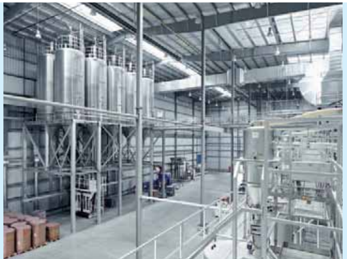
Indoor silos with finished goods for automatic bagging and palletising
