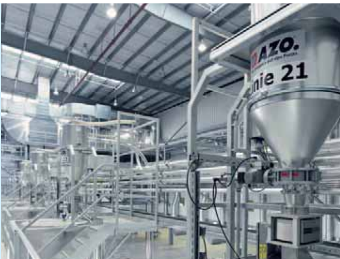
Feeding the day bins via receivers with subsequent metal separator
