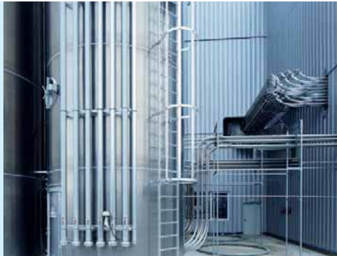
Silo fill lines with tank truck coupling
