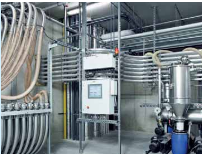
Manual coupling station for setting the route from the outdoor silos to the compounding lines
