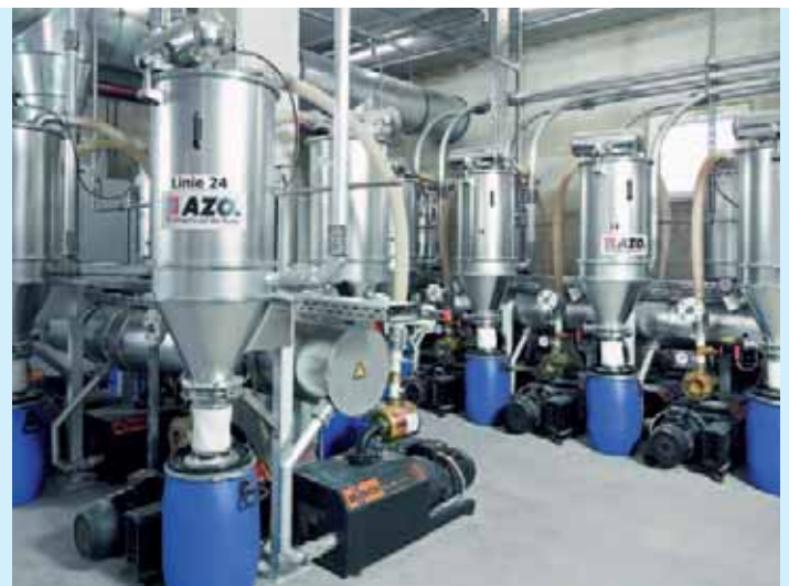
Vacuum pumps with upstream secondary filters in separate blower chamber
