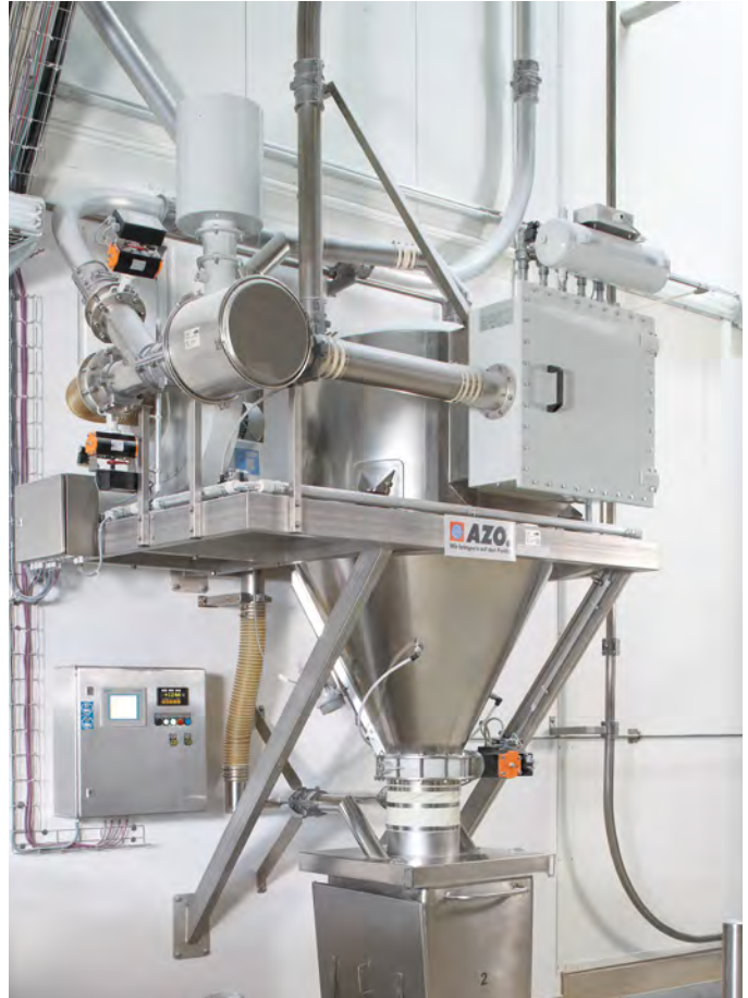
Vacuum weighing system with conveying scales for feeding the flour dispersing system
