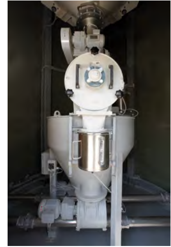
Skirt with cyclone screener and diverting hopper
