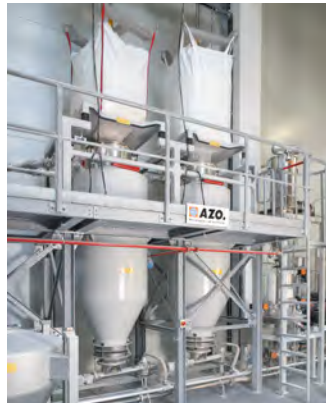
Big Bag discharge into buffer hopper
