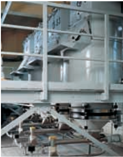
Bag dump station with bag cleaning
