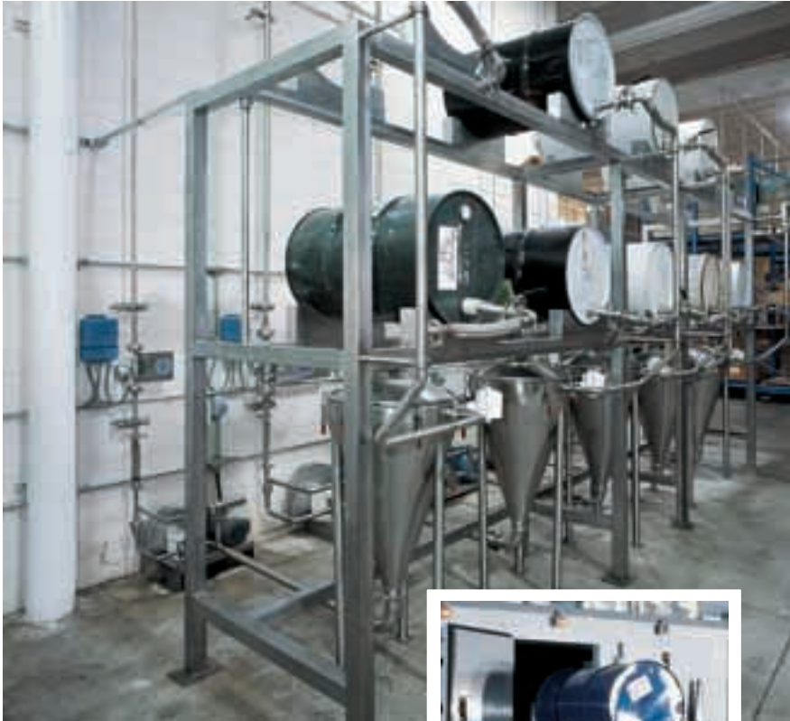
Feeding liquid minor ingredients supplied in drums
