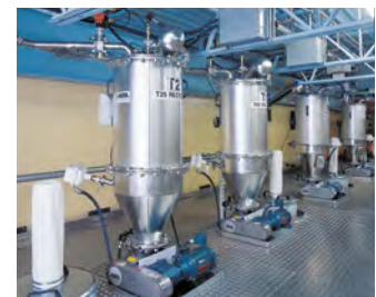
Pneumatic feeding into downstream processes
